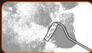
phase II: Apply the first coat of Diamento with irregular moves of a string roller.
