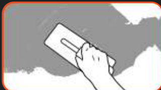
phase II: Apply a coat of Industrial Rust mixed with the Rust Activator.
