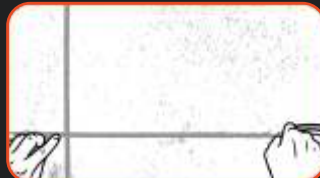
phase III: When the surface of Decorative Concrete initially dries, the tape which imitates rustications can be adhered.
