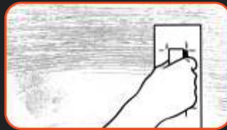
phase III: Model the pattern by dragging a brush trowel over the plaster.
